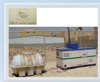
Kirloskar Generator Powering a Telecom site of ASACO
