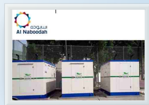
Site Installation at Al Naboodah with Kirloskar 500kVA Generating Sets.
